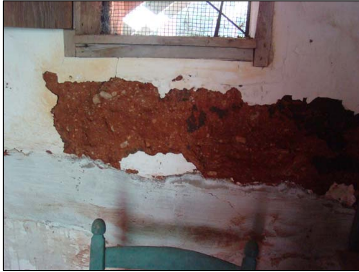
Figure 98. Interior wall showing some plaster loss inside the dairy/kitchen. (Photo: Author)
