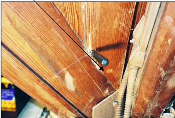
Figure 127. The screwdriver illustrates how soft the wooden roof trusses had become due to extensive termite damage. (Photo: Cummings and McCrady Architects)
