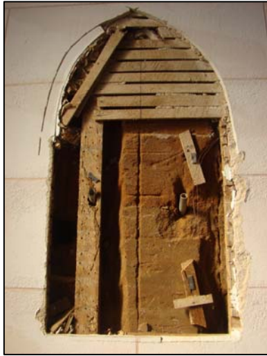
Figure 136. Area on north wall where a plaque used to be showing how modern conveniences have been installed through the pisé walls. (Photo: Author)
