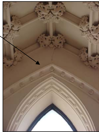
Figure 121. Arrows point to cracks due to weakened structure. (Photo: Author)
