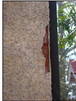
Figure 100. Closer view of area of pebble dash loss (about six inches in length) (Photo: Author)
