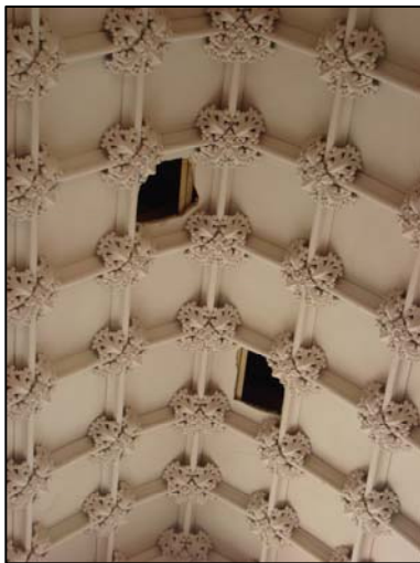
Figure 122. Holes cut in the Chancel ceiling to inspect and monitor termite damage. (Photo: Author)
