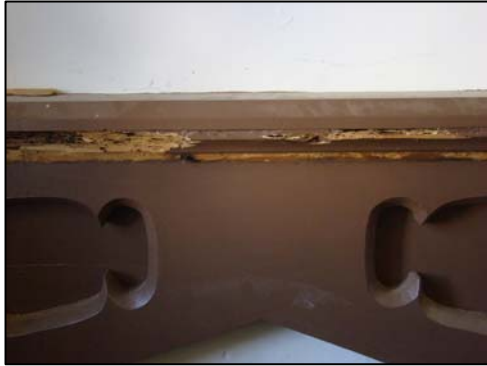
Figure 112. Termite damage on the mantle in Sacristy. (Photo: Author)
