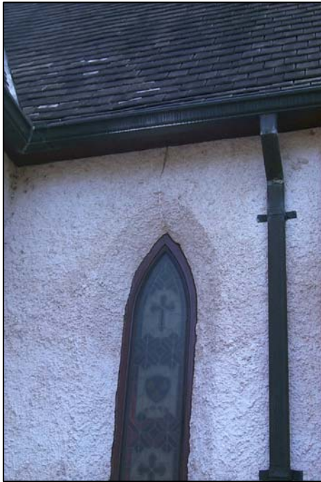
Figure 132. Cracking on the exterior render due to excess stresses from termite damage. (Photo: Cummings and McCrady Architects)
