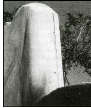
Figure 15. Same wall as in Plate 7 repaired with a new compatible stucco. (Photo: Lauren B. Sickels – Taves)
