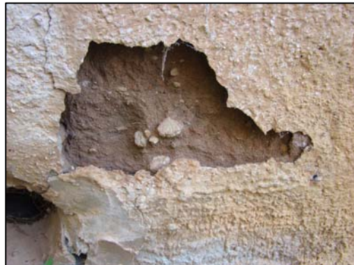
Figure 84. A closer view of the pebble dash loss where some of the earth has also deteriorated. (Photo: Authot)
