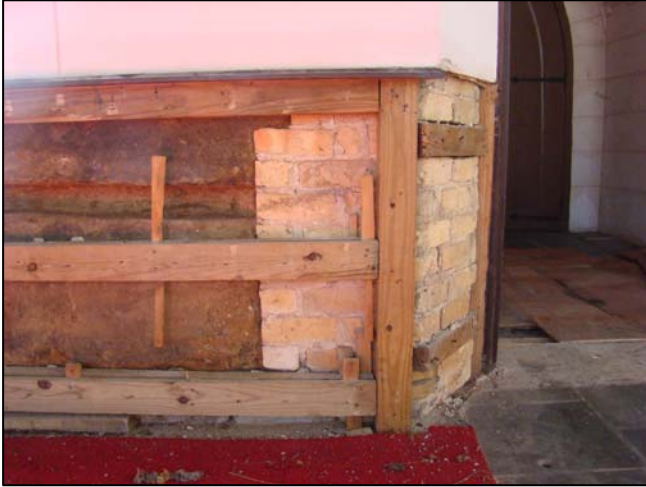
Plate A21. Brick repair made near the porch entrance on the south elevation. (Photo: Author)
