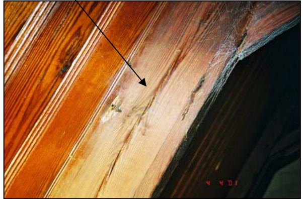
Figure 126. Cracking and separation of wood in roof truss due to termite damage. (Photo: Cummings and McCrady Architects)
