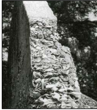
Figure 14. Damaged tabby wall with previous cement repairs at top. (Photo: Lauren B. Sickels- Taves)
