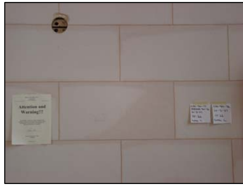
Figure 119. Holes cut in plaster to monitor termite damage. (Photo: Author)
