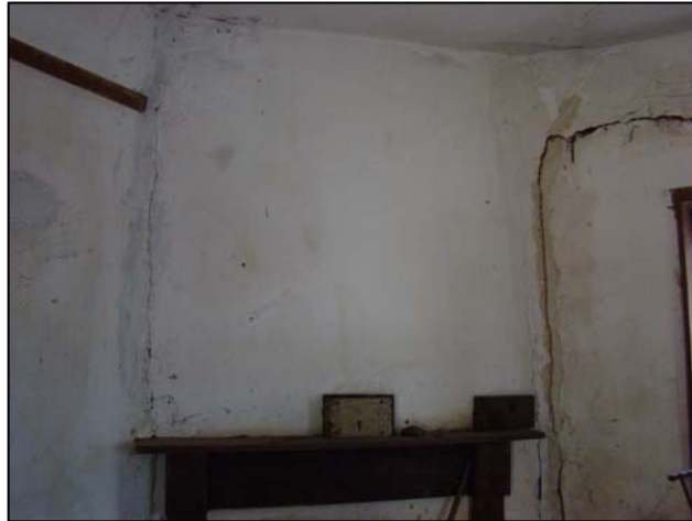
Figure 103. Large crack in the plaster of the loom house where a live oak's roots have disrupted the eastern wall of the structure. (Photo: Author)
