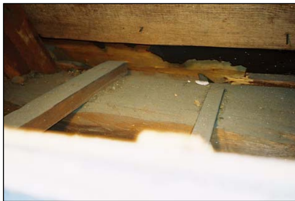
Figure 131. Another view through the hole cut in the Chancel ceiling reveals a wooden member that used to be a solid piece of wood. (Photo: Cummings and McCrady Architects)
