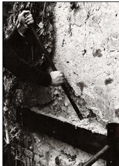
Figure 96. A cob wall being repaired and filled in with temporary shuttering. (Photo: John and Nicola Ashurst)
