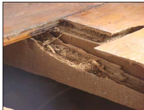
Figure 117. Severe termite damage on floorboards under choir area. (Photo: Author)
