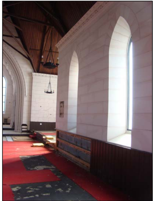
Plate A22. Concrete block repair made after the collapse of a portion of the south wall in 1974. (Photo: Author)
