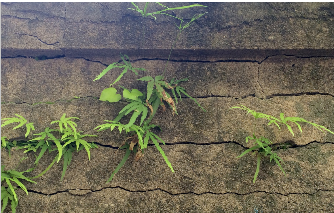
Figure 25. Detail of biogrowth in the horizontal cracks
