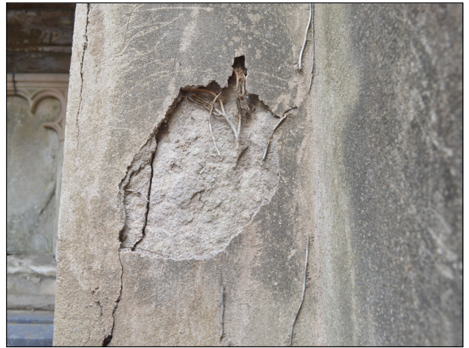
Figure 9. Staining and vines present on the east tower, vines have caused delamination, bulging and stucco loss.
