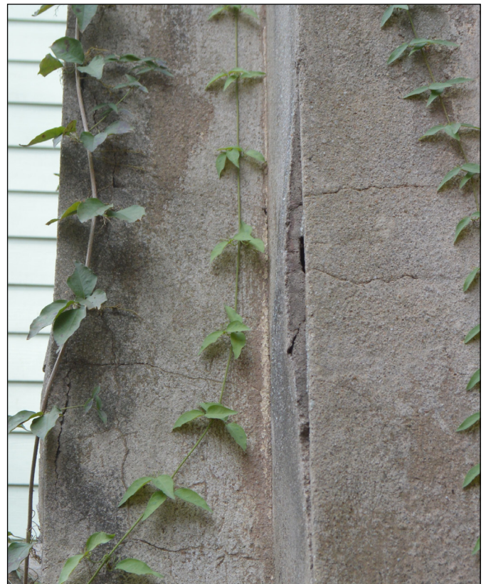
Figure 5. Bulging and delamination of the stucco.
