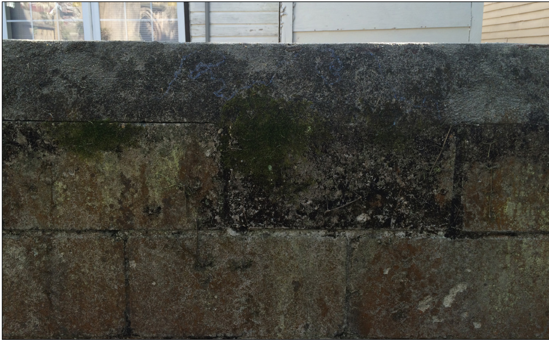
Figure 20. Staining and biogrowth on the east wall.
