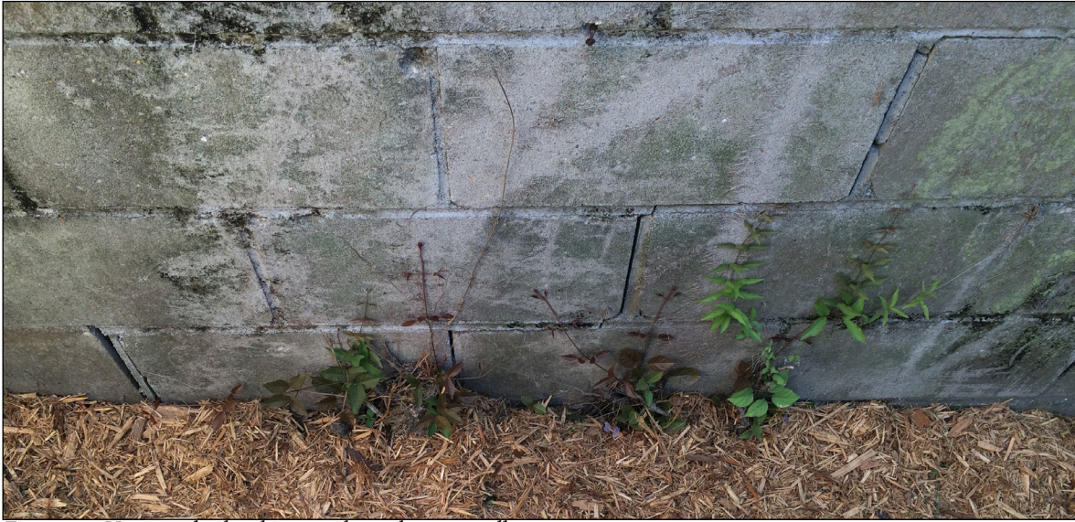
Figure 19. Vines and other biogrowth on the east wall.
