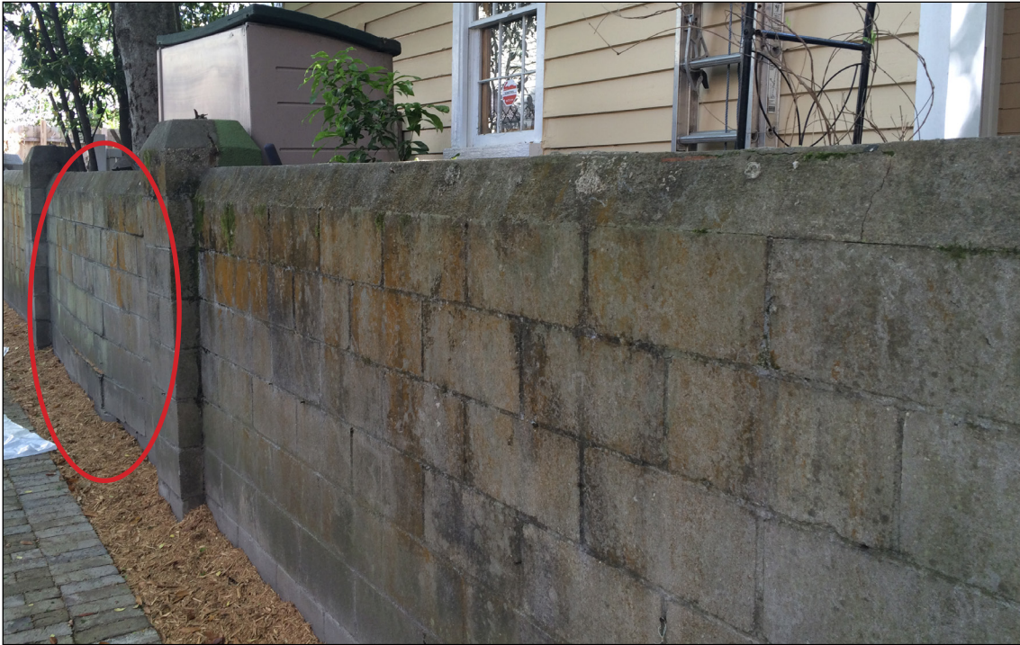
Figure 21. View of the east wall with bowed section
