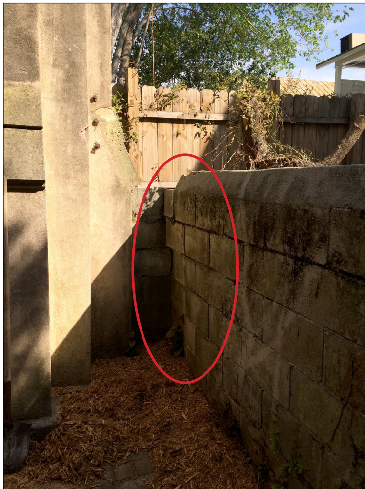
Figure 22. Bowing in the northeast corner
