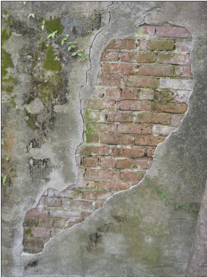
Figure 14. Area of Delamination
