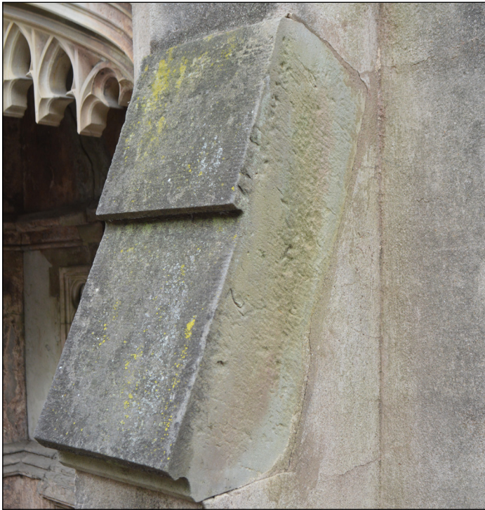
Figure 8. Staining and biogrowth present on the buttress
