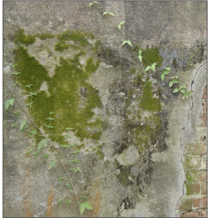
Figure 15. Moss and vines growing on the north elevation
