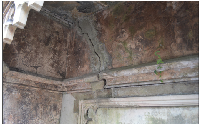
Figure 12. Major crack on the interior of the monument.
