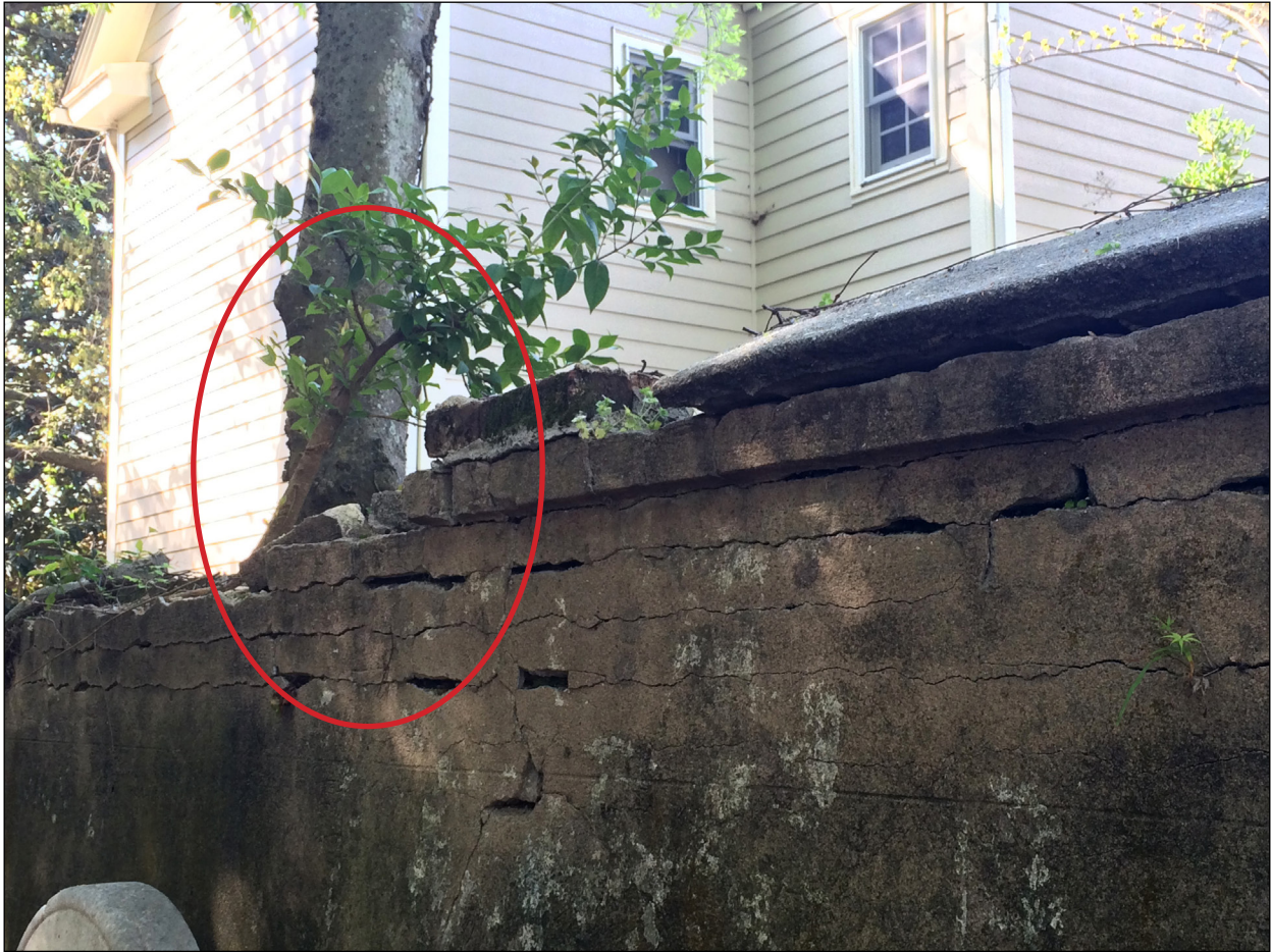
Figure 24. Horizontal cracks, biogrowth, and staining on the west wall. The small tree is growing from the top of the wall.
