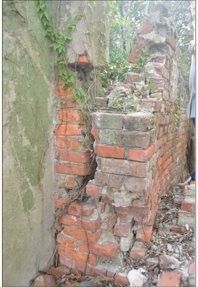
Figure 7. The crack in the west buttress from the north side of the monument
