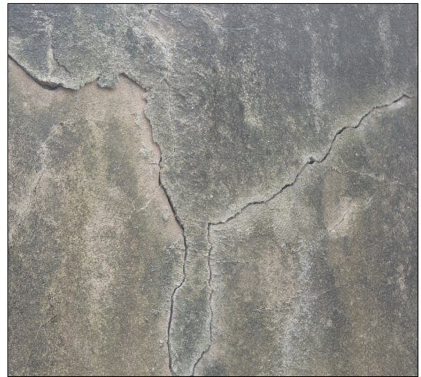
Figure 16. Area of delamination and poor repair.
