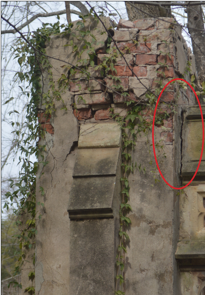
Figure 4. Leaning of the tower to the left with the broken connection between the stucco and brick and the stone.
