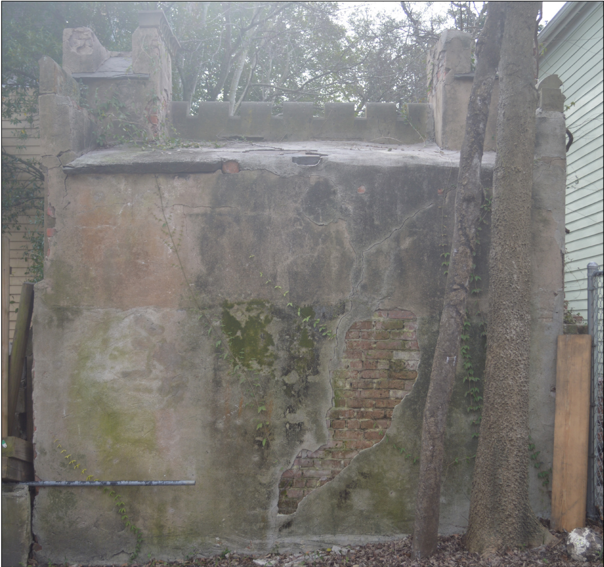
Figure 17. Displacement of the monument.
