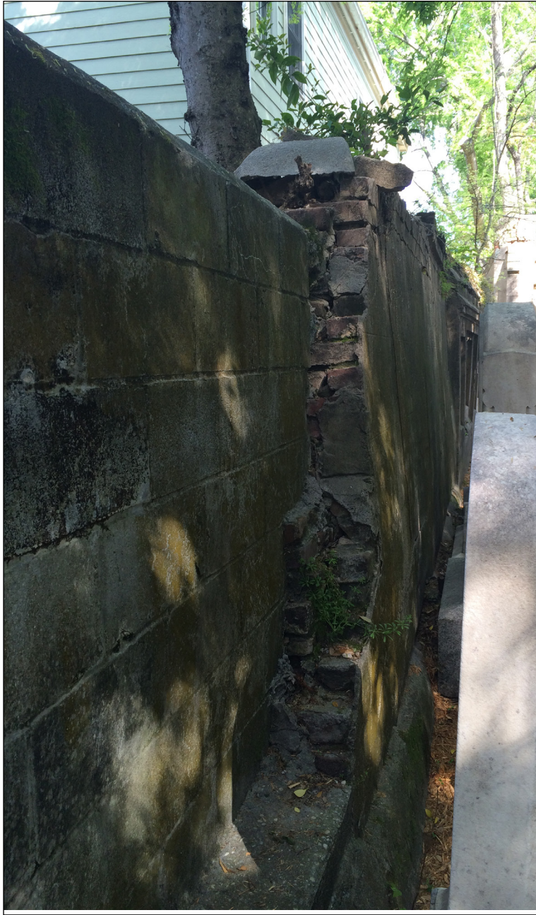
Figure 23. View of the stuccoed masonry and CMU sections of the west wall. Biogrowth and staining is visible on the CMU.
