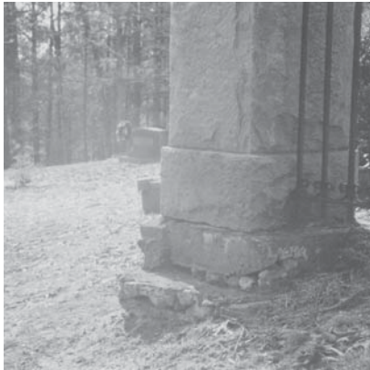
Deteriorating foundation at Calhoun family plot before repair
